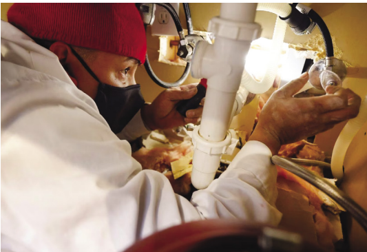
(BOTTOM) Contractor Giovanni 'Geo' Marino of Baker Brothers Plumbing repairs a broken water pipe under Joe Ellery's kitchen sink.
